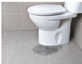
Fix leaking Toilet Immediately
